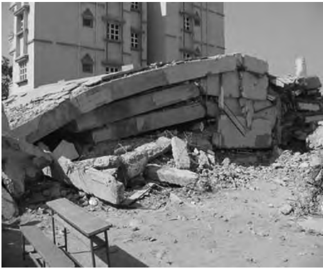
▲ Figure 2. Pancake collapse of a reinforced concrete (RC) frame building in the Bhuj earthquake, 2001. Photo: Earthquake Engineering Research Institute (EERI, 2002).
